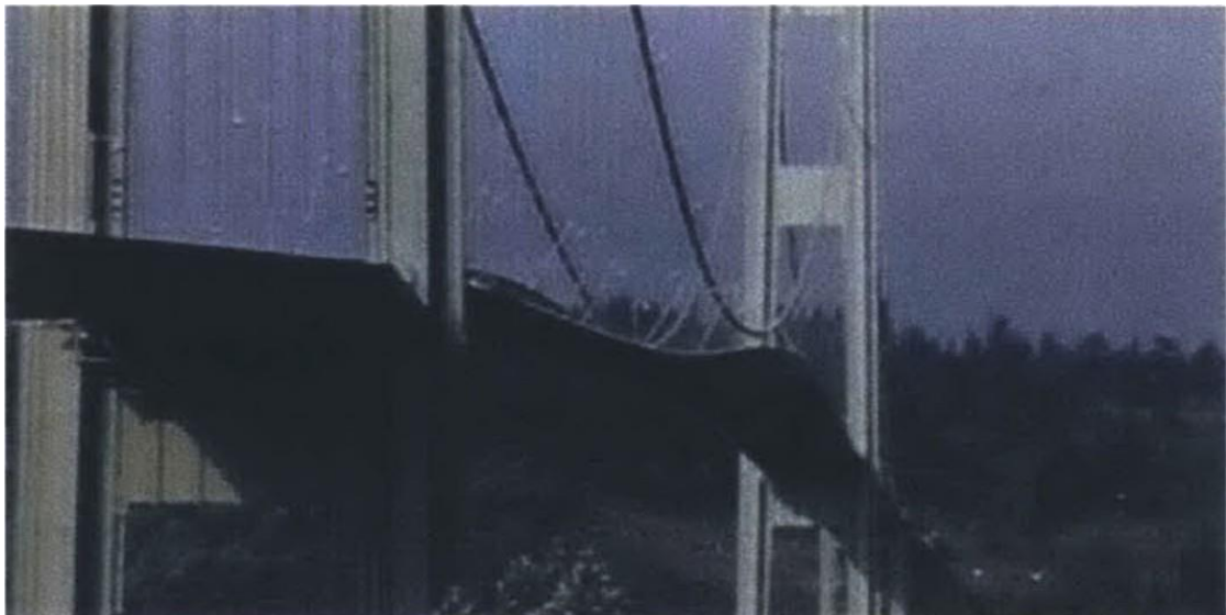
Figure-1. Resonance-Induced Severe Deformation and Eventual Collapse of the Tacoma Narrows Bridge.
